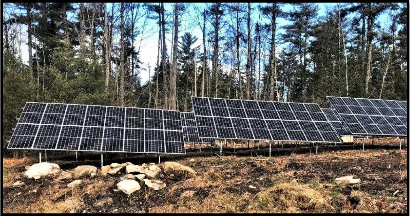
Figure 1: The array consists of 94 panels mounted on six frames on the hillside behind Sugar Hill's Town Garage.
